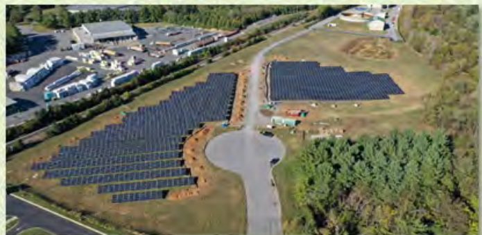
Above: Aerial view of the final solar array—Frederick County's first solar project. The project was funded through a $2.4M grant from MDE's Energy Water Infrastructure Program.
